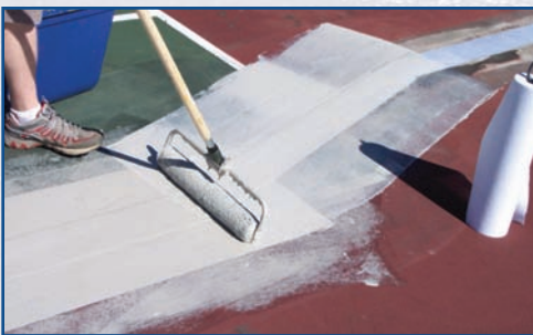
RiteWay Crack Repair System: Laying down micro sealant tape and stress mat.
